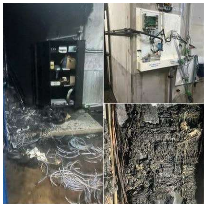
Draveil (Essonne) 1 st /2 nd July: the electrical system at the leisure centre set alight
