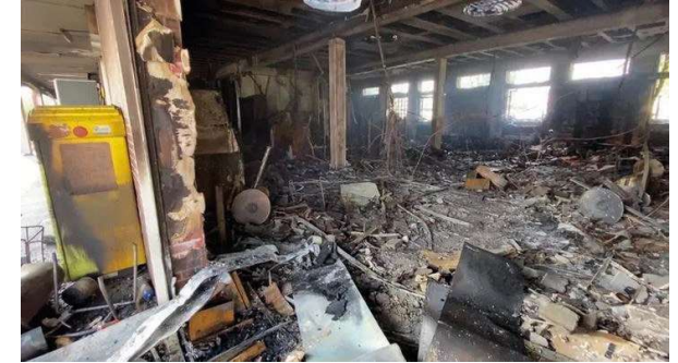
Poitiers (Vienne), 30 th June: police station of the Coronaries district in ruins
